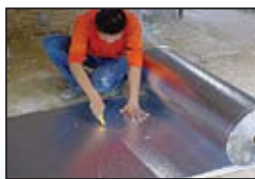
Step 1 Measure the width of the roof and by using blade cut the length accordingly.
