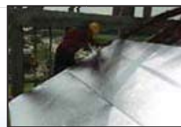
Step 3 Using self-tapping screw for light weight trusses or stapler for timber trusses to secure CoolMax™.
